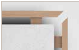
open miter joint
